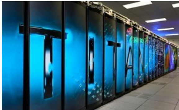
The Titan supercomputer has 18,688 GPUs
